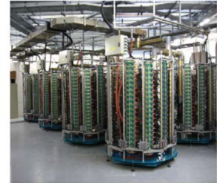
180 kW 350 MHz solid state amplifier, each column 45 kW (Soleil)
